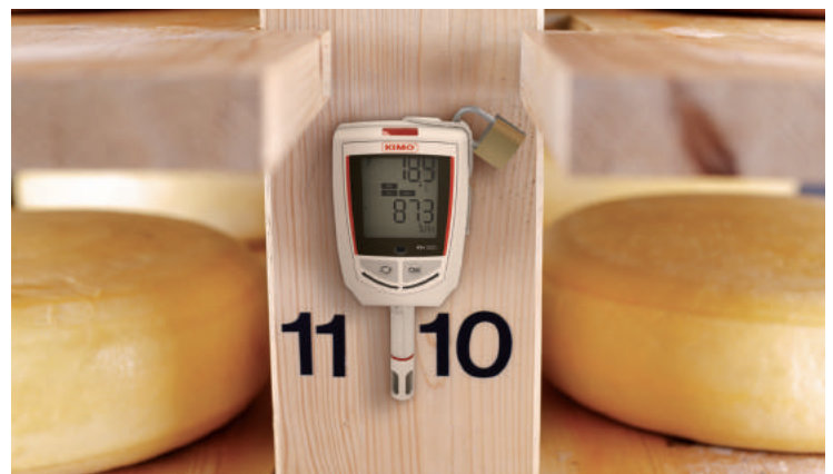
Relative humidity and temperature control in a maturing cellar using a KH 220 mounted onto a plate and secured with a padlock as part of a mapping process
