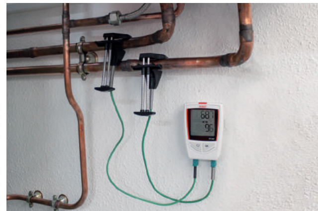
KTT 220 equipped with two clipped thermocouple sensors to control the domestic hot water network (DHW), mounted onto a wall plate
