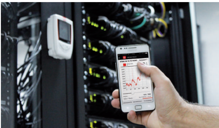
Control of climatic data from a data centre using the smartphone application
